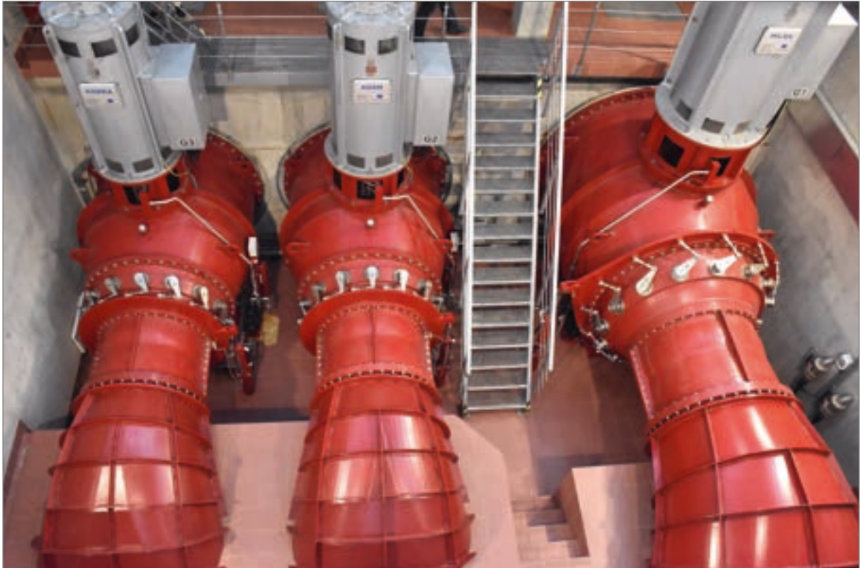
In the last two decades, state-of-the-art facilities have been built
