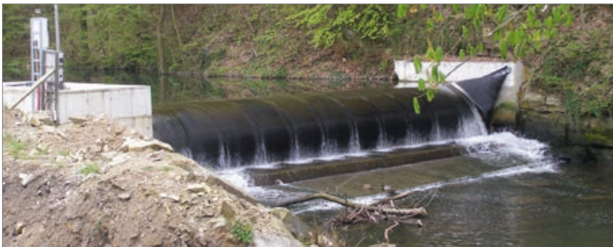
Hydraulic structures at SHPs significantly retain water in weir pools within riverbeds, contributing to water retention across the broader landscape
